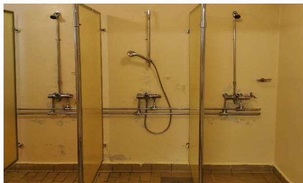
Figur 35: Fuktskader i garderober
